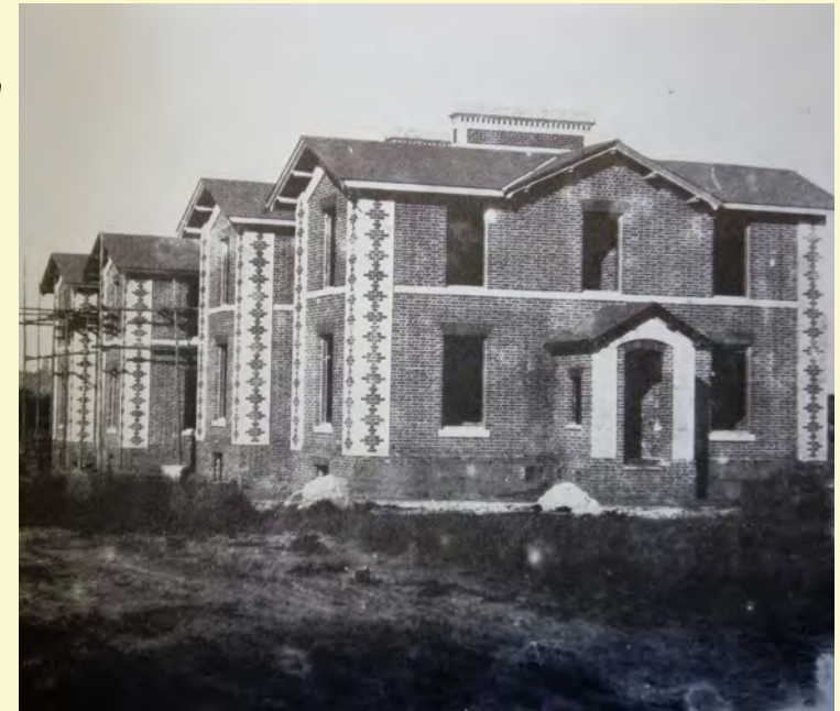
Houses in Burlington Road under construction in the early 1860s. The surrounding landscape illustrates the edge of town, undeveloped character of the area in the mid 19th century. (Ipswich Remembered 2, Suffolk Records Office, 1979 reproduced with kind permission of Suffolk Record Office, Ipswich branch).
