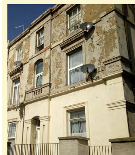
London Road: Buildings in need of general maintenance, with the repainting of the render required. This terrace also shows the impact of subdividing properties into flats there are a plethora of satellite dishes on the principal elevation and an inconsistent approach to replacing fenestration, with the above image showing several different types of window styles which erodes the integrity of the terrace.
