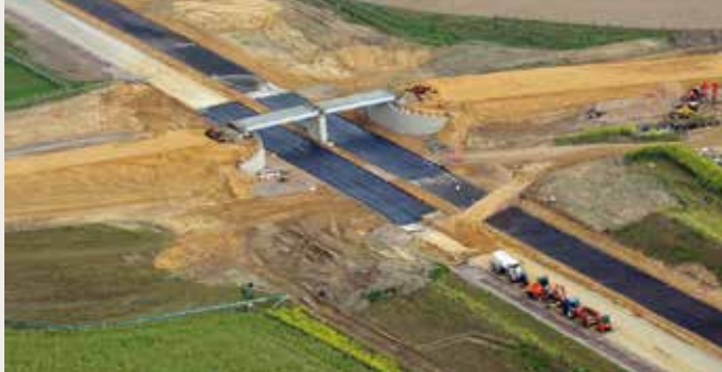
Left: Bell Farm track bridge and stabilisation, Norwich Northern Distributor Road Below: Greater Gabbard Wind Farm, East Coast
