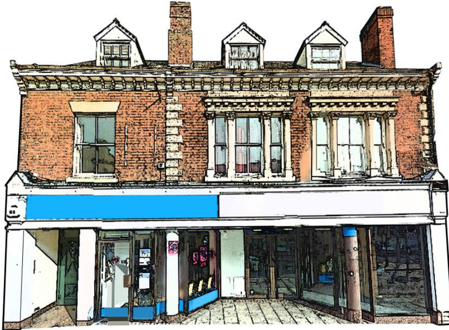
Fig 4 – An example of shopfront design which fails to reflect the overall architectural character of the building. The first floor shows a clear separation between principal and secondary elements, indicated by the quoins and the prominent windows, but there is no corresponding division of the fascia in this position. In addition, the large entrance opening visually undermines the principal part of the facade.
