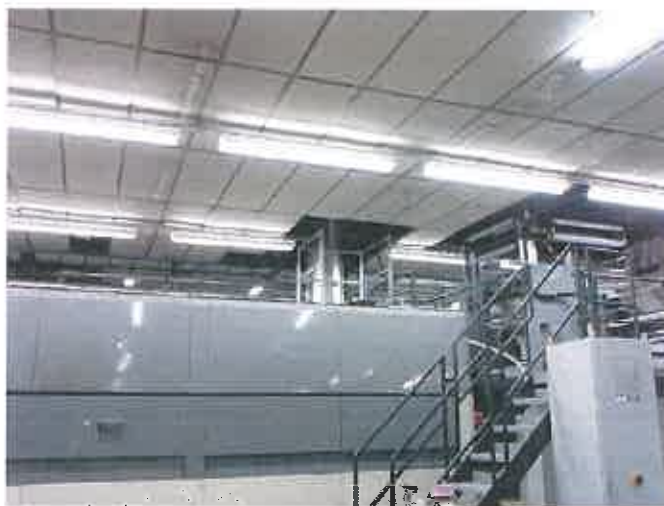
Stack showing test points
