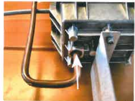
Figure 8 The pipe is assembled into the outlet of the meter
